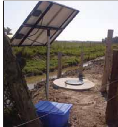
A solar-powered water system keeps livestock out of streams.
